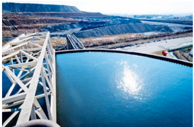
High-rate thickener for coal, 20 m in diameter
