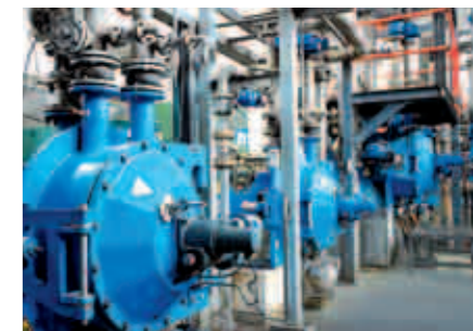
▲ LC refiner in the existing Xinya mechanical pulping fiberline.
