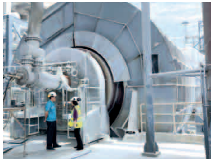
The lime reburning kiln has a capacity of 800 t/d. ▶
