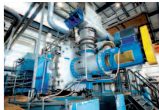
◀ Second-stage refining will include a HC refiner operated in atmospheric mode – similar to the existing Yinhe fiberline.
