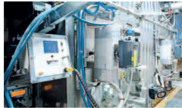
▲ The Iggesund boiler is one of the most automated in the world. Shown above are some of the combustion monitoring and air control systems.
